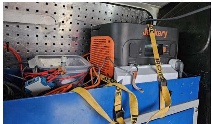
Fig. 4: Raspberry Pi, relays, connections to car battery and ignition, Jackery Explorer 2000 Pro with smart Zigbee socket and Starlink FHP dish power supply.
